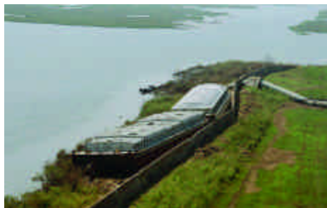
Barges washed up on Michoud's levee during Hurricane Katrina, damaging the I-wall.
