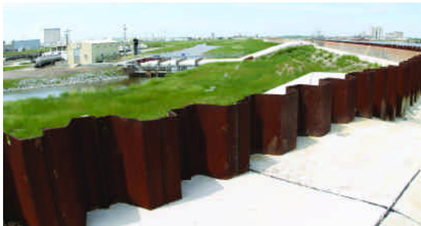
Near Michoud's pumping station, the Corps of Engineers' contractor drove 80-foot sheet pilings to reinforce the I-wall and poured flowable concrete to prevent erosion at the wall's base after Hurricane Katrina.
